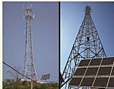
Solar Communication Station Power System
