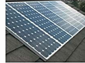
Roof Mount Solar
